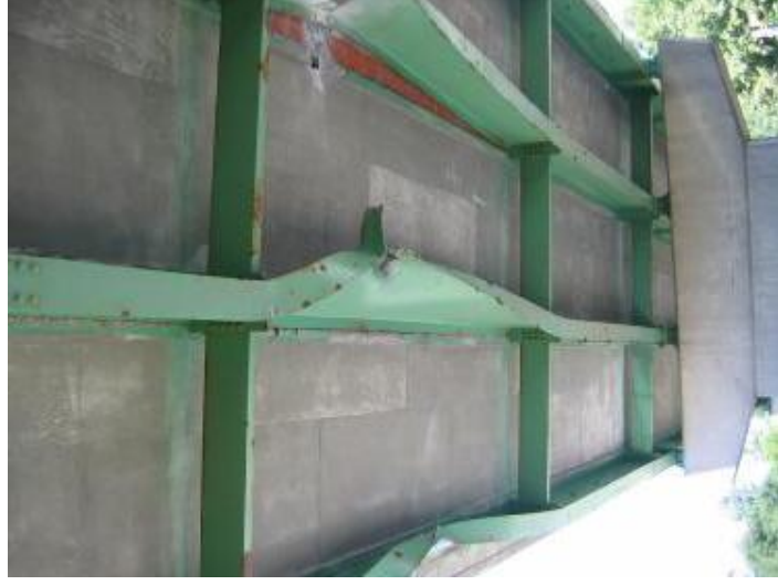
Hackett Road Bridge Hit - 2005
